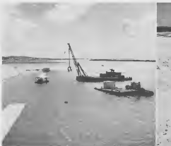
THE QUAY WALL, a section of which will be covered with banded concrete slabs, will be 350 meters long. Huge concrete monoliths are fabricated on the site, floated by barge to position and then lowered in place by a floating crane. The Barcadera Harbor has a navigable depth of thirty-six feet. E MURAYA di waf, un parti di cual su vloer lo worde cubri cu e planchanan di concreto cu nan rand furá cu hero, lo ta 350 meter largo. Hokknanan gigantesco di concreto ta worde trahá na e sitio ey, ta worde poná ariba un lancha pa laba nan na un lugar y despues nan ta worde baha den awa door di un graa cu tin ariba un lancha.
